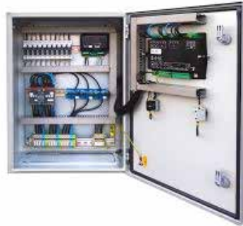
Automatic Transfer Switch panel
